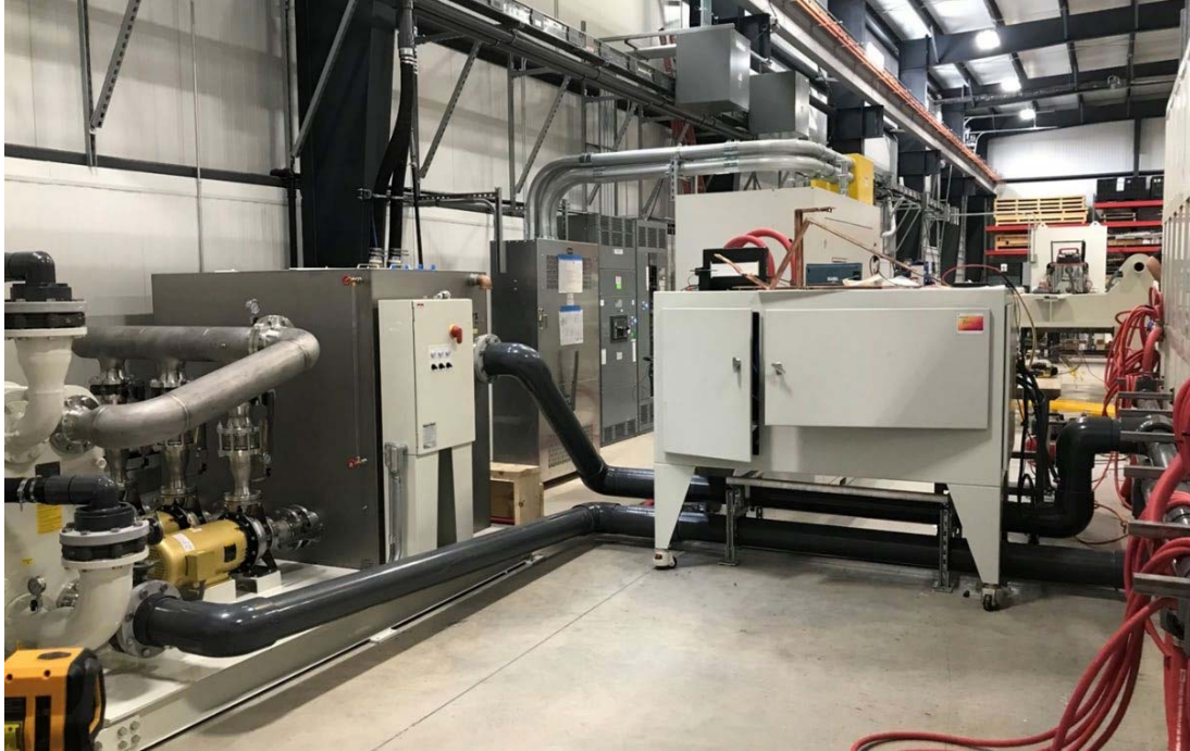
Figure 51. Picture of 1MW power supply connected to the tool along with the water supply with pump connected to the power supply and tool
