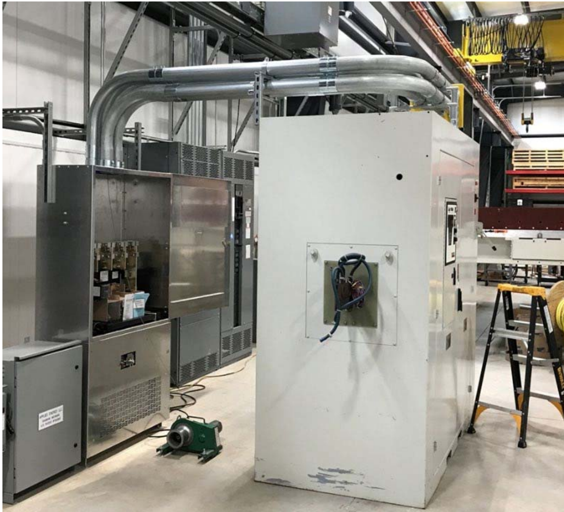
Figure 48. Picture of the 1MW 1 to 3 KHz induction power supply during installation adjacent to the large scale restraint.
